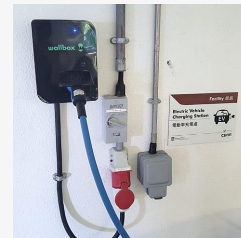
Electric Vehicle Charging Station in Faculty of Medicine Building, Sassoon Road Campus
