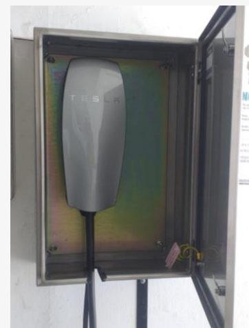
Electric Vehicle Charging Station
